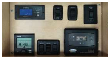
Convenient control center monitors capacities
